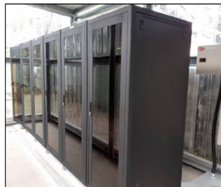
Storage Systems of MG2 and MG3
