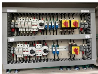
Switches of Solar Panel of MG2 and MG3
