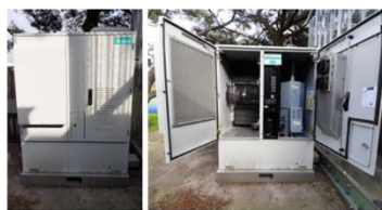
Hydrogen Fuel Cell
