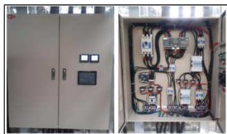
Switches of Interconnected System
